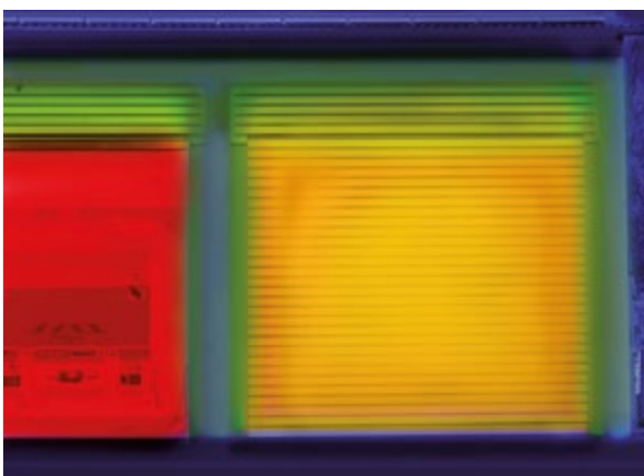
This thermal image of an ordinary roll-up door clearly shows the large heat loss to the outside.
